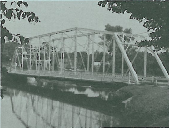
Photo 5. Washington Road Crossing over Fish Creek, Ionia, Mich. Single-span pin-connected camelback through truss, 1906.
