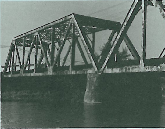
Photo 9. Pere Marquette Railroad Crossing over Raisin River, Monroe, Mich. Two-span riveted Warren through truss with verticals, 1911.
