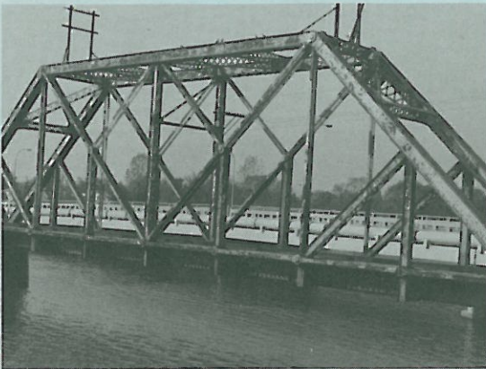
Photo 7. New York Central Railroad Crossing over Raisin River, Monroe, Mich. Three-span (only one is shown) pin-connected Baltimore through truss, 1910.
